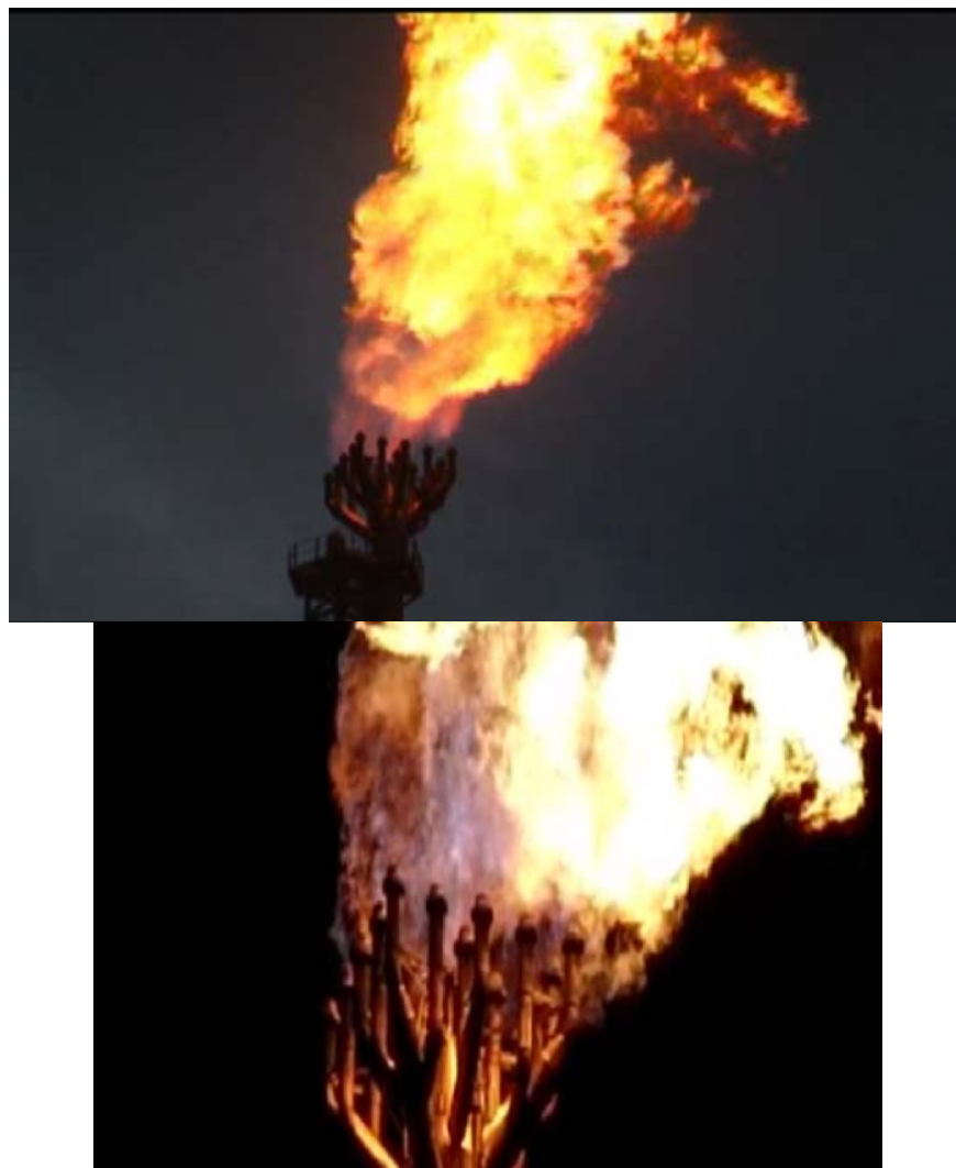
Figure 1 - Elevated multi-tip HP air flare firing natural gas
